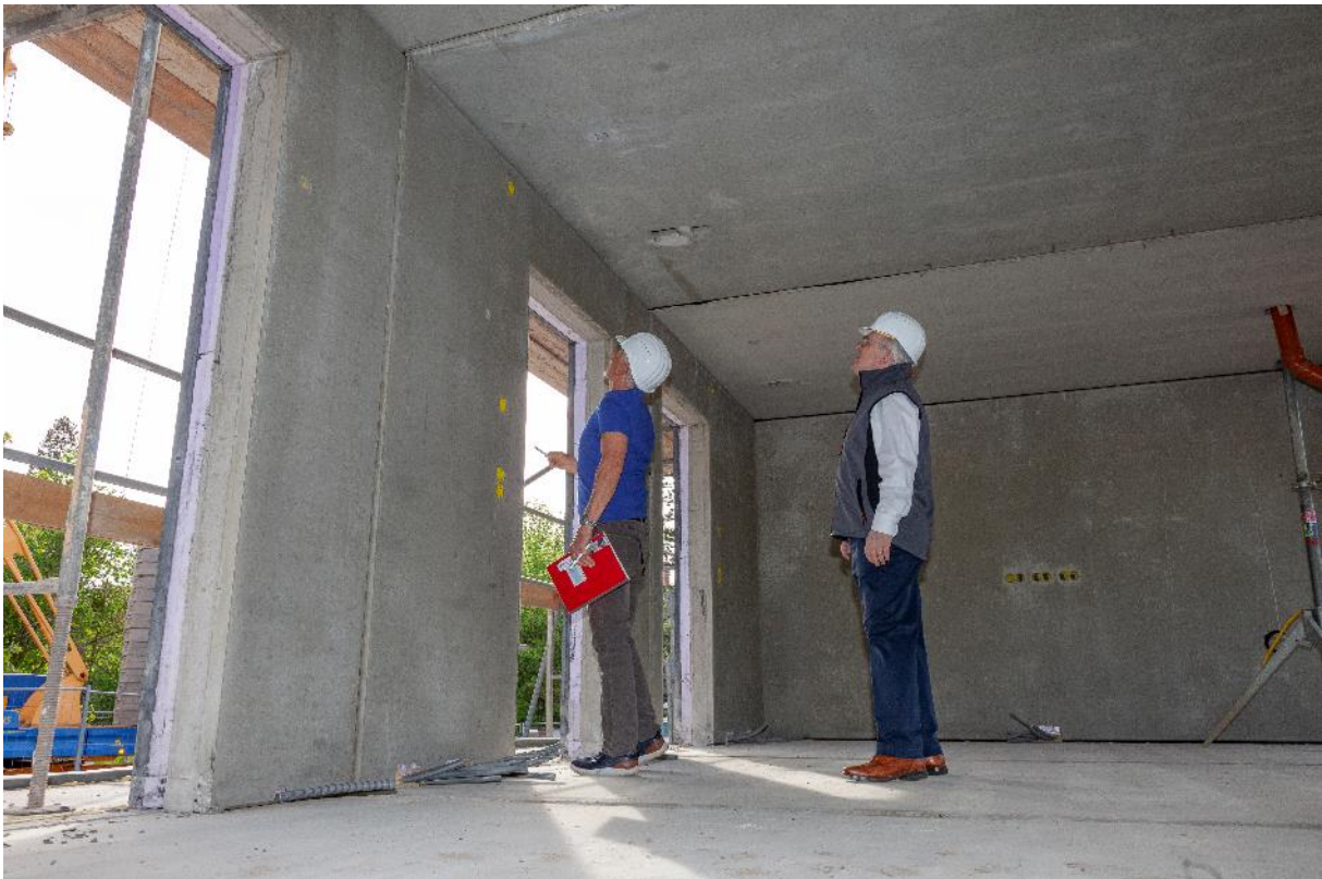
3: Last check before the successful partial acceptance of the BOX: Michael Molitor and Manfred Curbach (from left to right). © Stefan Gröschel, IMB, TU Dresden
